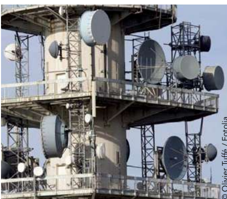
Telecom - Data infrastructure
