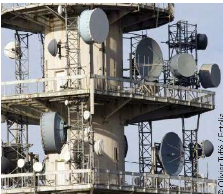
Telecom - Data infrastructure
